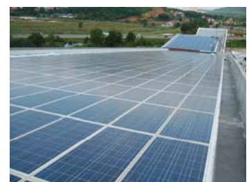
92kWp PV system PTM-ZEO
