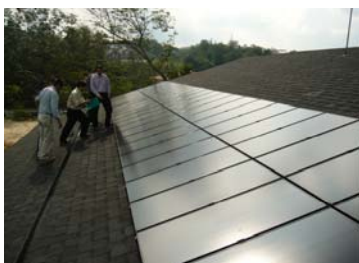
4kWp PV system Damansara Country Heights
