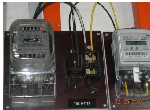
Direct feed – TNB and PV meters are located side by side
