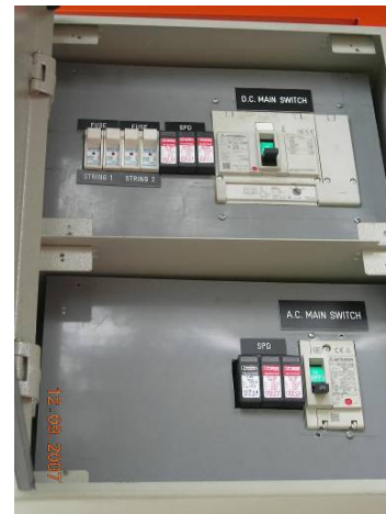
Control box (SPDs, MCCBs and switches)
