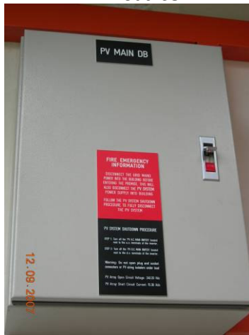
Safety labels are in place
