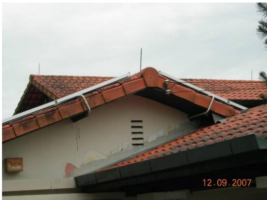
No drilling to the roof. Cables are properly sealed inside conduit and done neatly.
