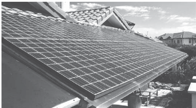
Source: Kota Damansara, 3.15 kWp, Selangor, Malaysia.
