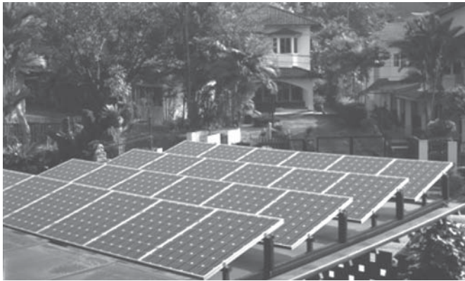
Source: Bukit Damansara, 4.2 kWp, Kuala Lumpur, Malaysia.
