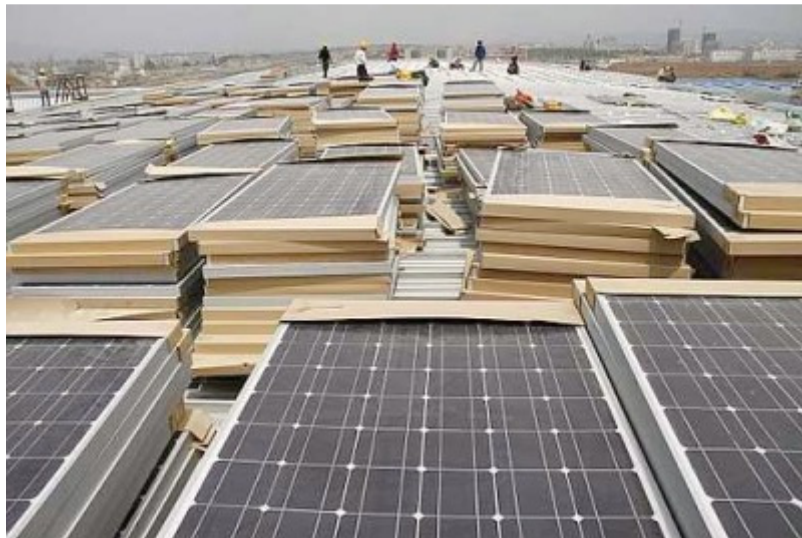
Harnessing free power: Workers installing solar panels on the rooftop of the Nanjing South Railway Station in Nanjing, Jiangsu province, China. Production of solar power is expanding worldwide. China, for instance, has more than doubled its target for solar power capacity to 50 gigawatts by 2020.
